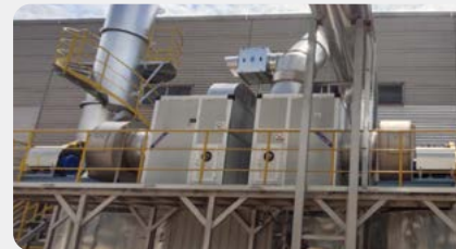
VOCs oxidizer waste heat recovery system
