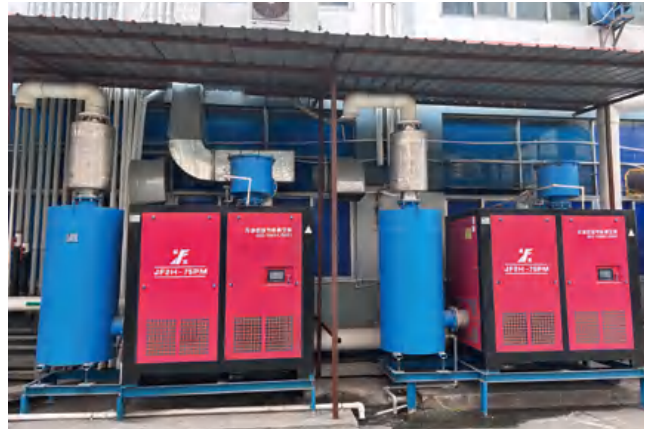
New Ventilation Facilities
