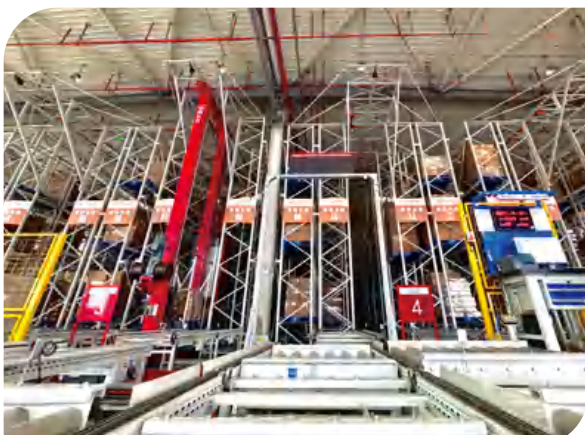
Three-dimensional Intelligent Warehouse
