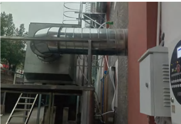
New Facilities for Managing Exhaust Gas Emission
