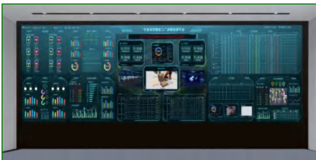
Dashboard of Situation Command Center
